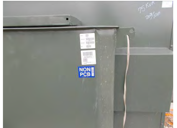
Photo #34 View non-PCB label observed on pad-mounted transformer at 14225 West 67 th Avenue (Parcel 39-063-02-001).
