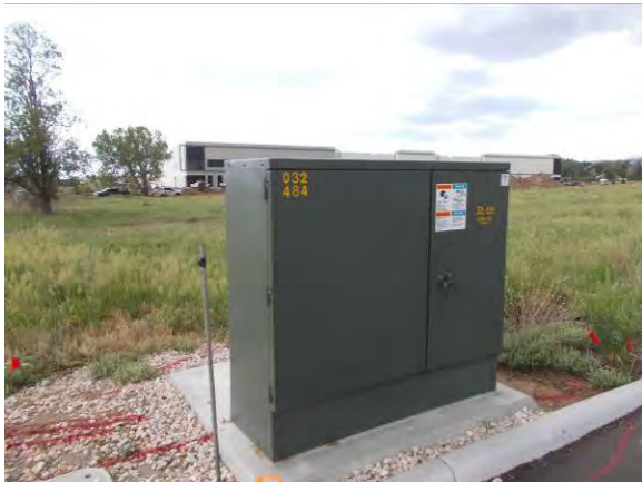
Photo #33 View of pad-mounted transformer observed near northeast corner of 14225 West 67 th Avenue (Parcel 39-063-02-001).
